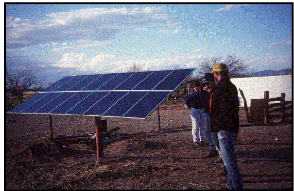
Figure 1. Typical program installation: PV water pumper in Rancho Jeromin, Aldama, Chihuahua.
